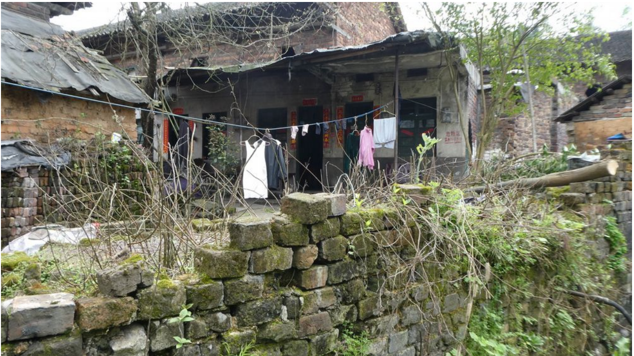
A simple run-down house in a terrace of single storey houses.
