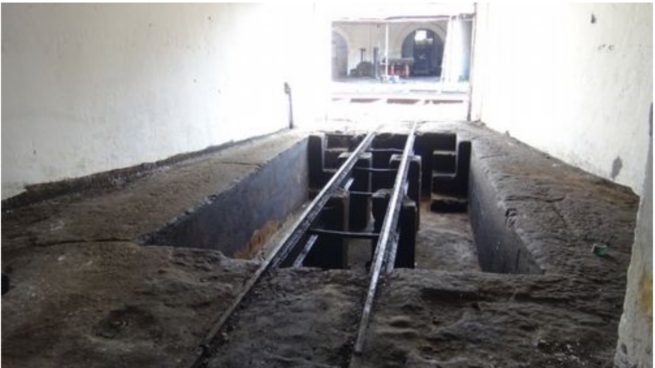
Steam era loco servicing pit could still see use for diesel loco repair.
